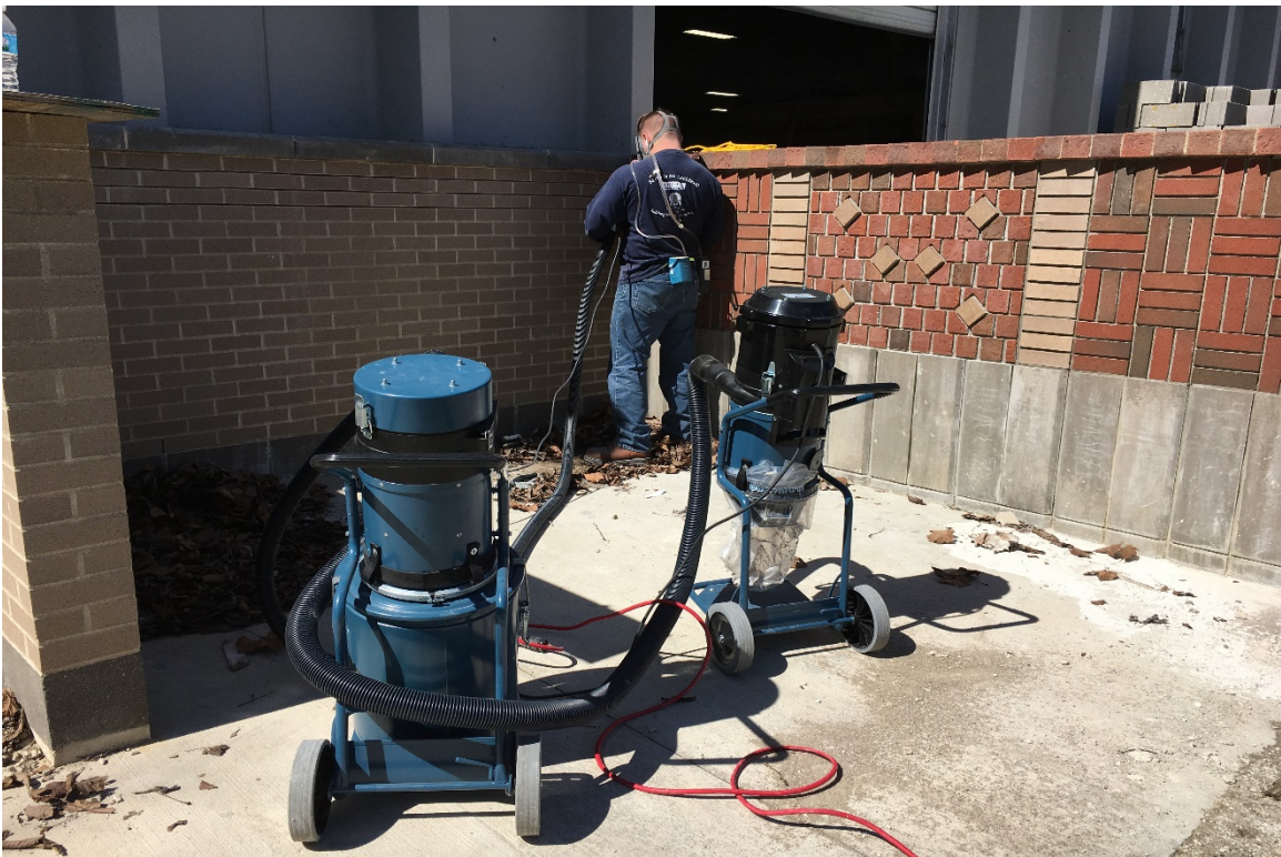
Figure 3 - Pre-separator (left) and vacuum cleaner (NIOSH photo)
